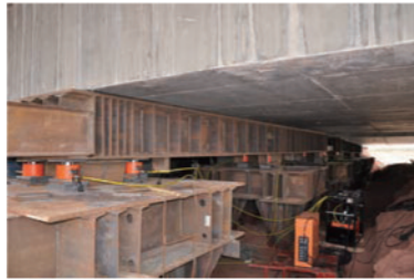
24 EAGLE PRO ESL series hydraulic cylinders with an EAGLE PRO electric hydraulic pump lift a bridge into position
